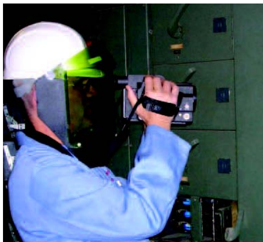
Infrared thermographers look for hot spots that could indicate loose connections and other electrical problems.
